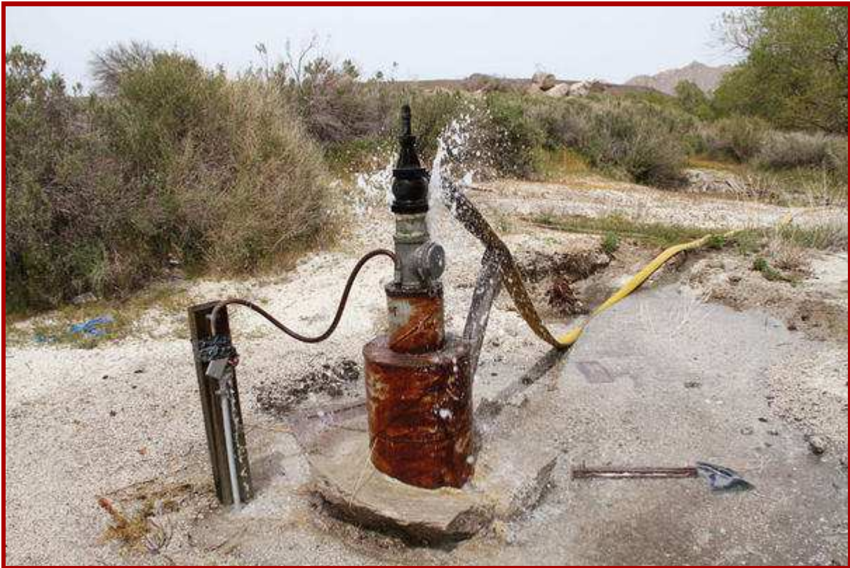
Fig. 7 Jacumba Water District's well head, flowing under artesian conditions on April 17, 2010.
